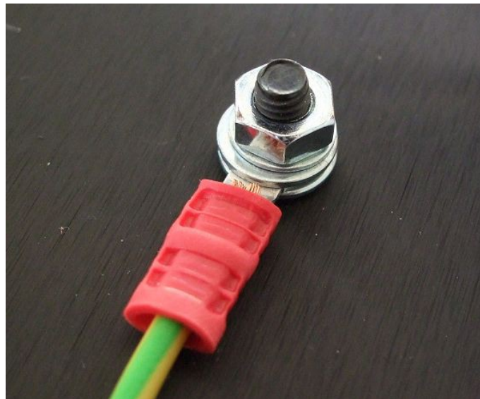
An earth bonding point using an M4 screw, two washers, two toothed washers and nut. The earth wire uses a crimped 4mm ring terminal.
